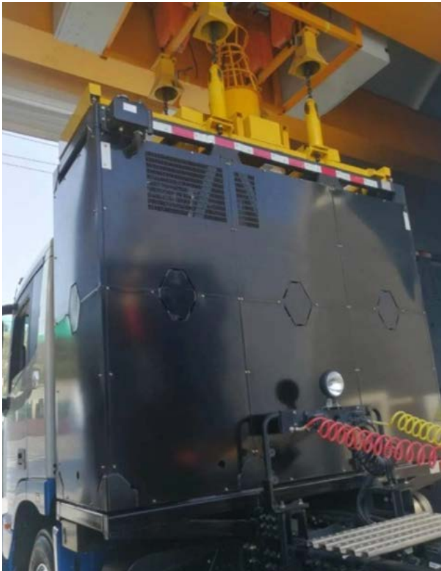
Figure 29: Battery location in this project.
